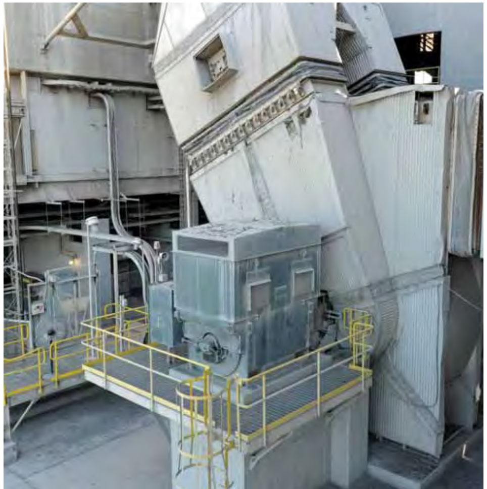
The kiln-induced draft (ID) fan is powered by a 5,000 HP WPII Baldor•Reliance large AC motor. The ID fan is a central element in the clinker production process as raw meal is fed into the kiln and sintered.
