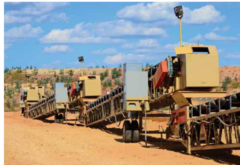
Baldor’s System-1 group facilitated the order processing, packaging and preassembly of the Baldor equipment for the 21 grasshopper transfer conveyors. Because of the number of gearboxes, motors, pulleys and bearings required, Goodfellow managers say the System-1 team saved them valuable time.
