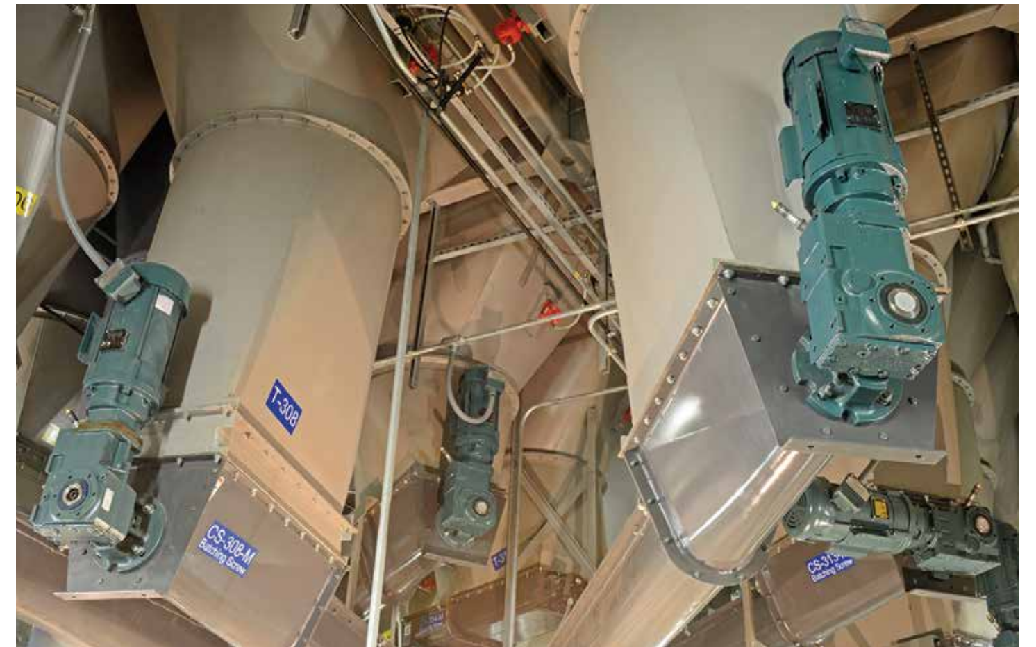
Screw Conveyor Corporation chose to use Baldor•Reliance explosion-proof motors and Baldor•Dodge Quantis Right-Angle Helical Bevel (RHB) reducers on the 15 batching screw conveyors. The motors are rated Division 1; Class I, Group D; and Class II, Group F & G, ensuring safety and reliability in a hazardous environment where combustible dust is present all or some of the time. RHB units were selected for their greater torque density in a compact housing.
