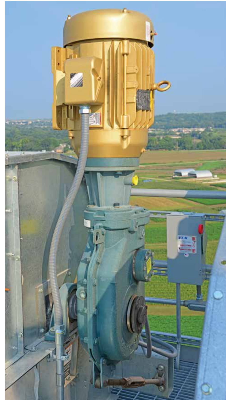
For the bucket elevators, SCAFCO chose Baldor's Dodge Motorized Torque-Arm II® (MTA) gear reducers, a heavy-duty, right-angle beltless Torque-Arm, for its ease of maintenance and its compact, space-saving design. It also selected Baldor•Reliance® Super-E® premium efficient motors, which run cooler and longer with better reliability than any other industrial motor.
