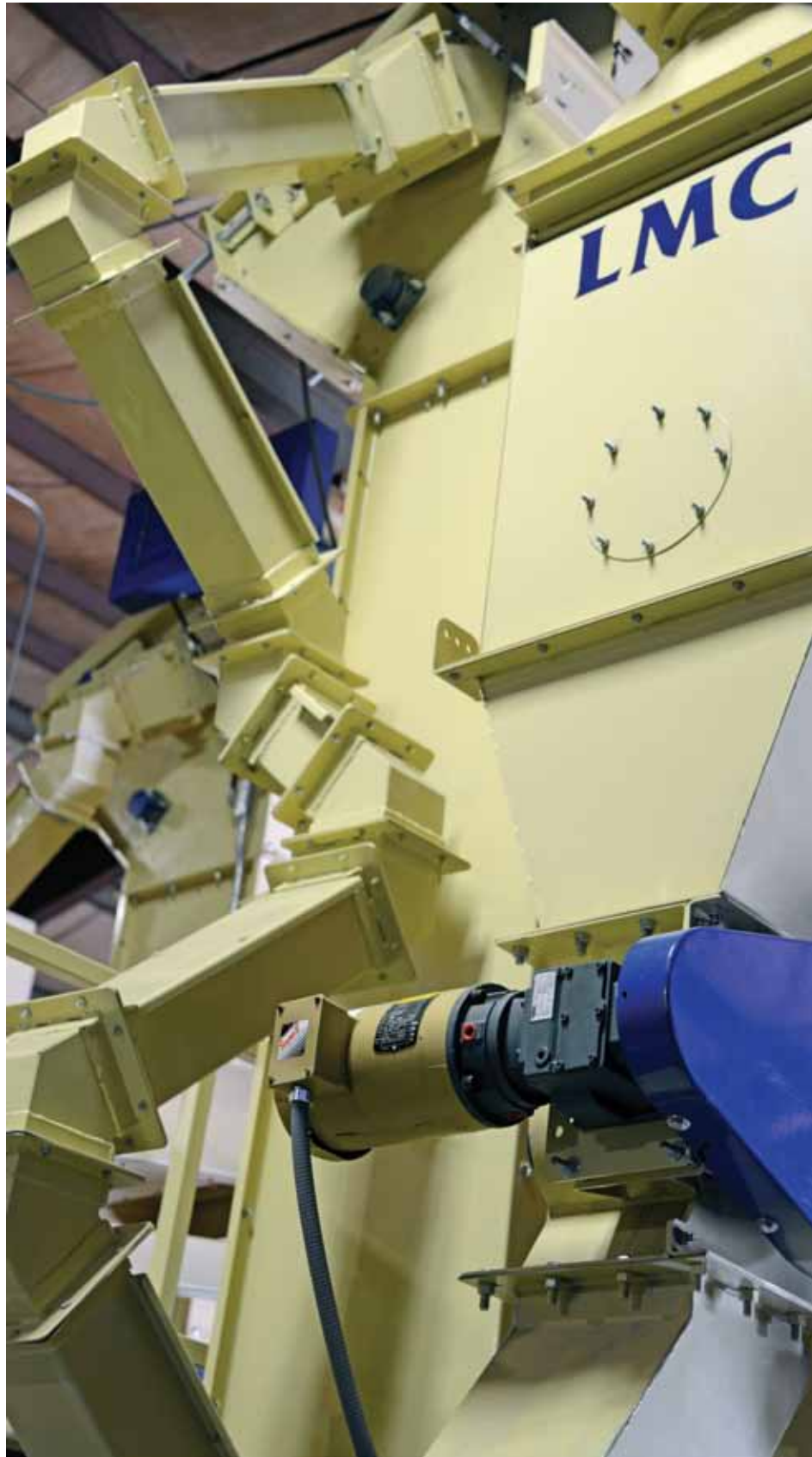
LMC officials say they chose Baldor as their global partner because they can rely on them for the whole gamut of electrical and mechanical products. For example, this Baldor•Reliance® motor and Baldor•Dodge® Quantis® reducer package installed on an LMC aspirator, a piece of equipment that uses air flow to separate materials.
